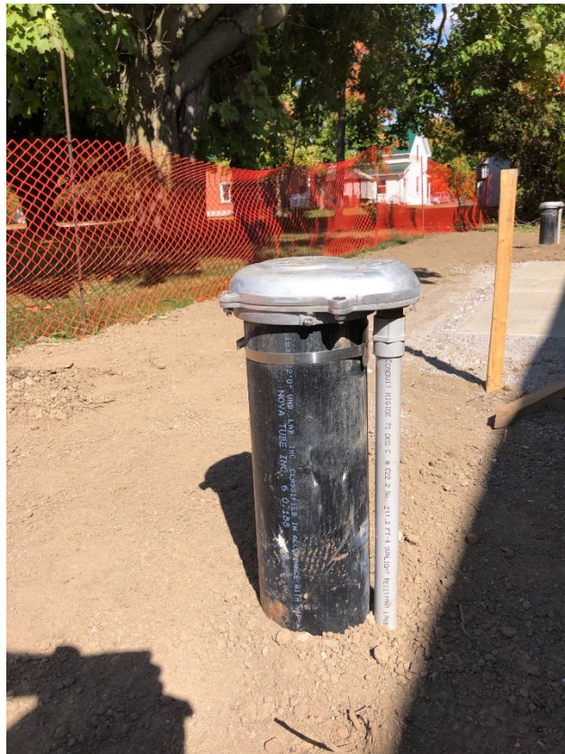
View of drinking well installation
