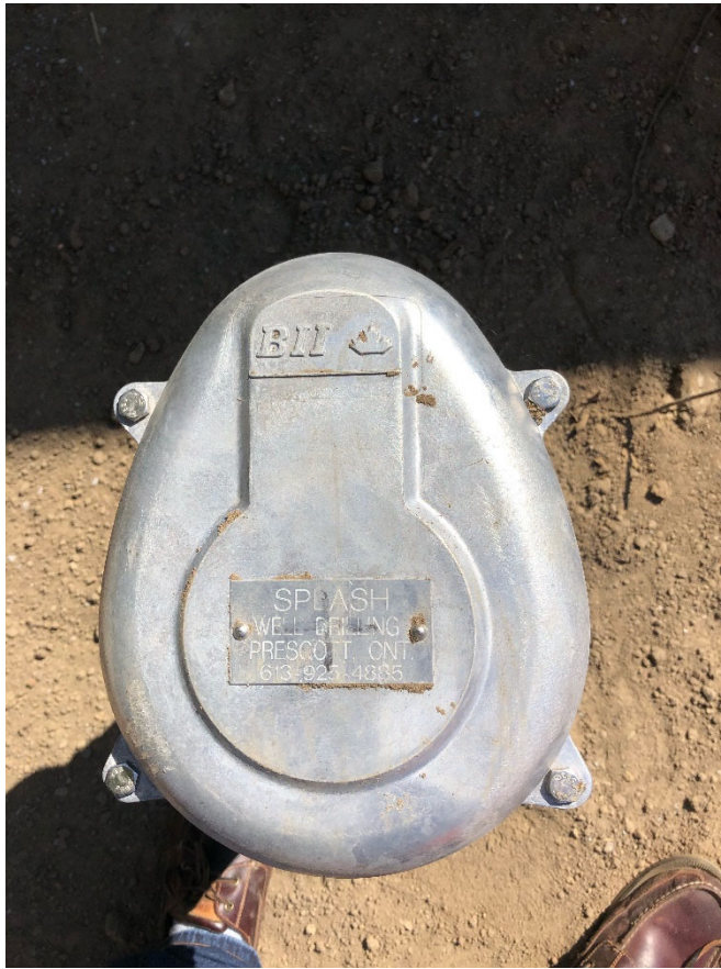
Well cap including details of drilling company
