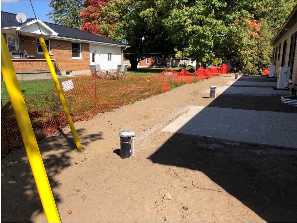
32 David Street, individual unit drinking well installations
